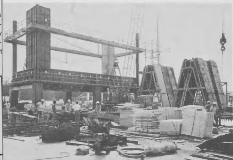
Shown here is the precasting of refractory slabs on the steel walls (at right) which are then installed in sections to form the furnace wall.
